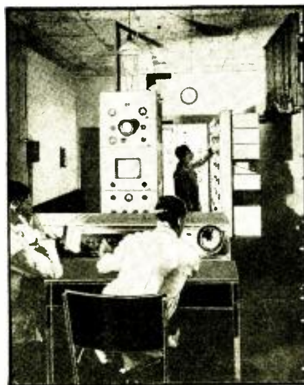
Control room and amplifier racks for the Baird installation at Alexandra Palace. Note the monitor cathode-ray image tube on the control desk (right) and the acoustically treated walls and ceiling. The Baird installation is alternated with the Marconi-E. M. I. system. Each station is usually on the air one day while the other is silent.
